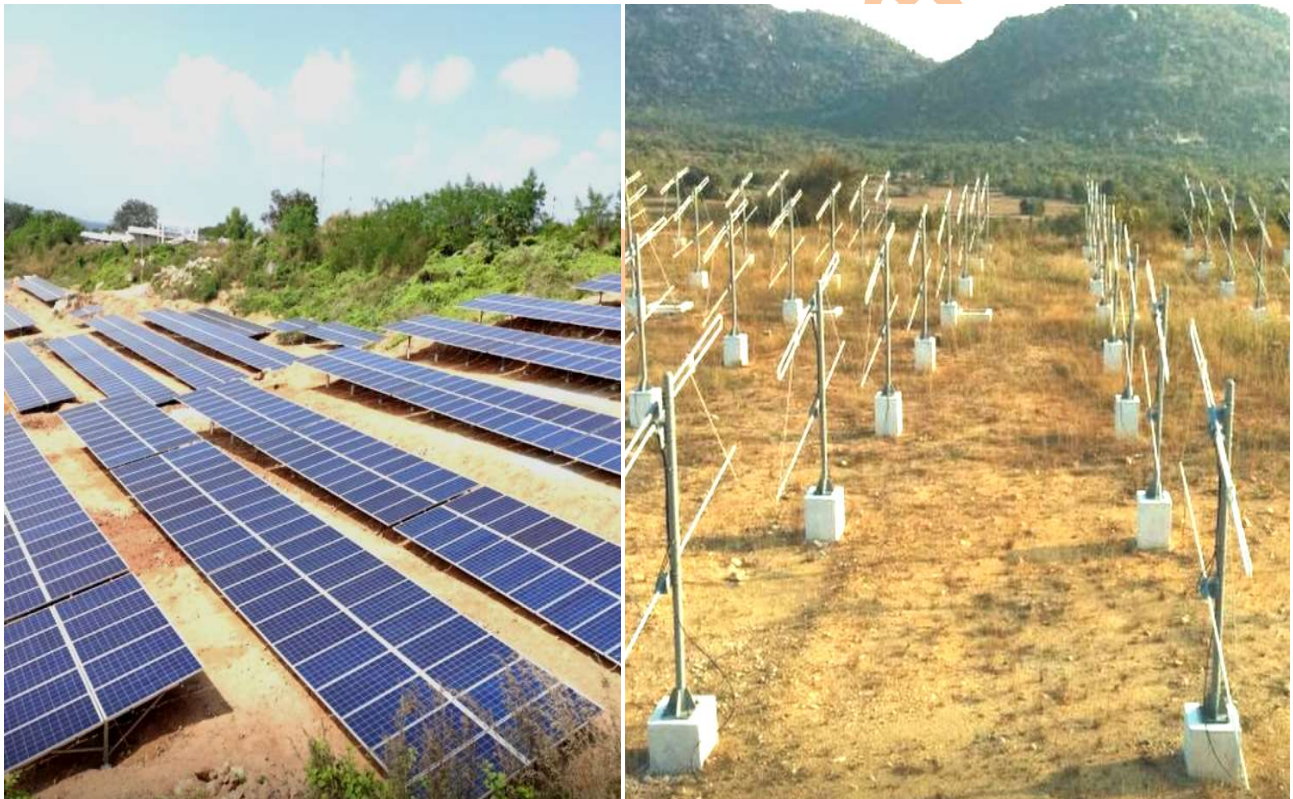
Solar panels and Radio communication System at NARL
